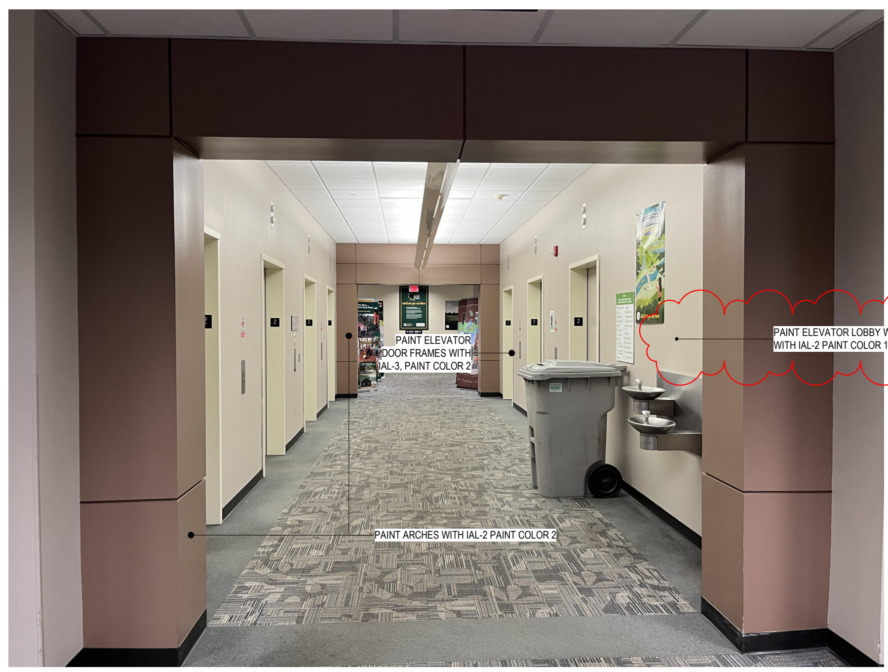
7 ARCHES AND DOOR FRAMES TO RECEIVE PAINT COLOR 2 REF: 1/A-101 SCALE: NTS
